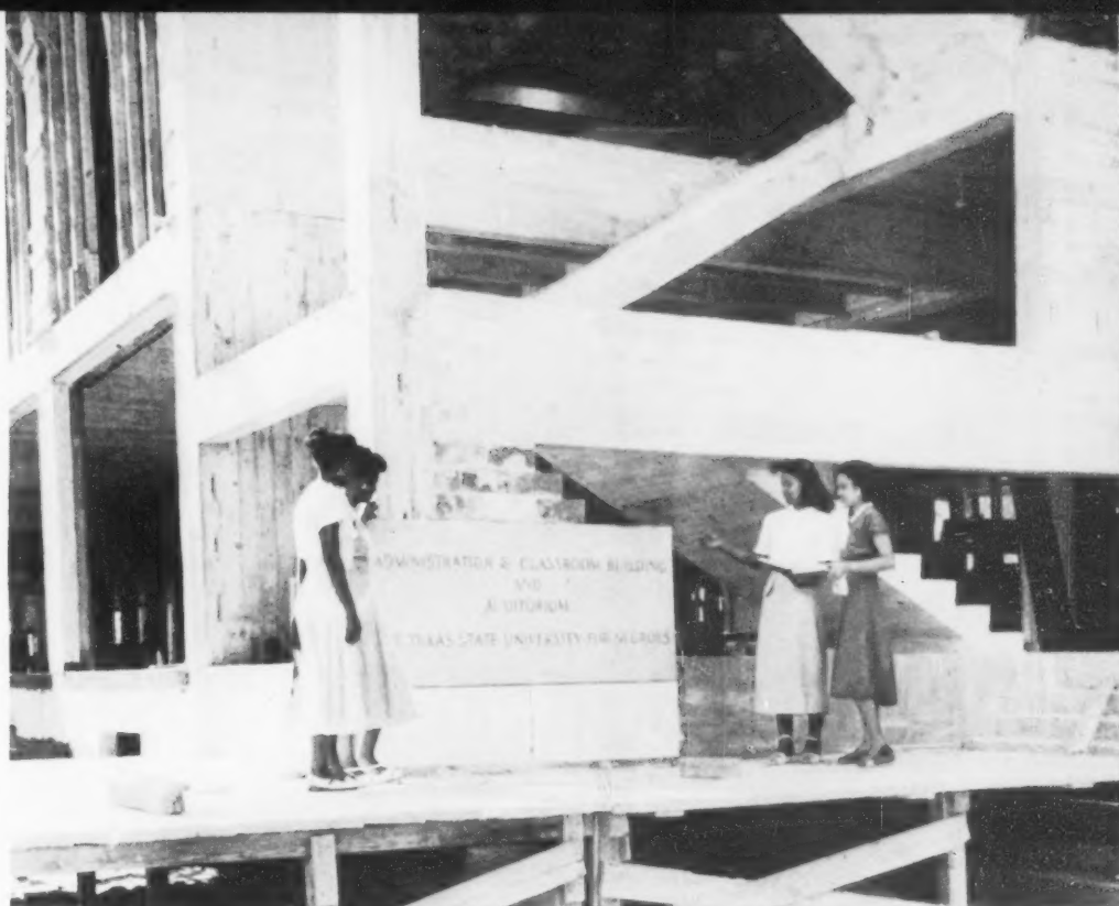
New Texas State University for Negroes is being built at Houston from ground up at cost in excess of $10,000,000 as result of U. S. Supreme Court decision in Heman Sweatt case ordering equal college facilities for Negroes.
